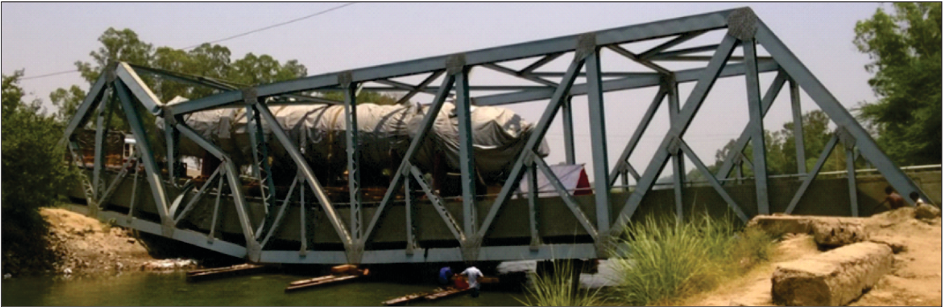
Fig. 1 : View of the Collapsed Bridge Over Canal
