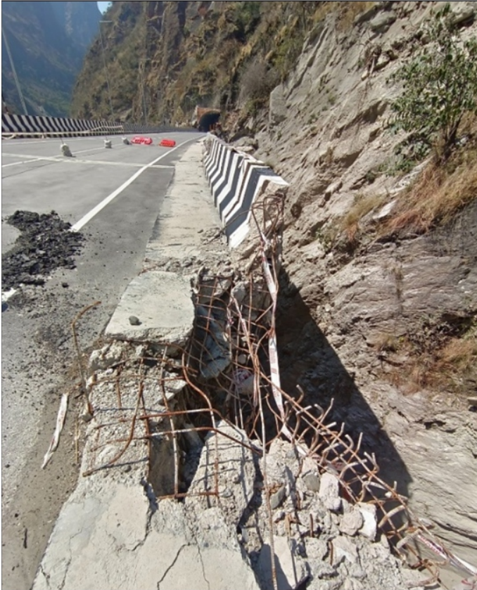
Photo 2 : Damage due to Boulder hitting the deck Note : Elevated bridge edge is very close to hill side. A big boulder crashed on to the parapet and rolled on to deck slab.
