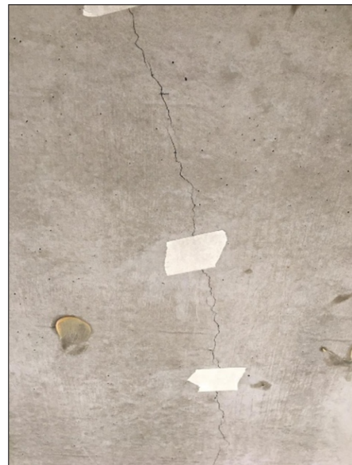
Photo 2: Closed View of Crack
