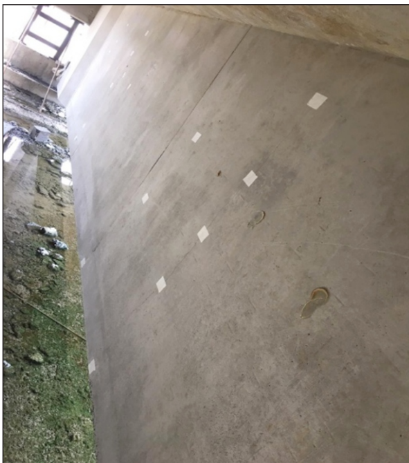
Photo 1: Elevation of Girder showing cracks
