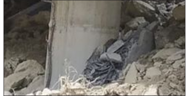
Enlarged view of pier completely broken in two pieces. Removal of debris could trigger further slide.
