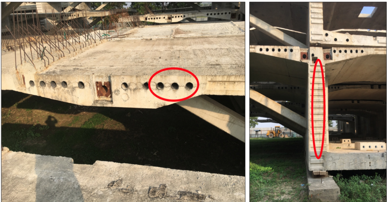
Fig. 4 : Left : Central horizontal cracks in top flange; Right : Central vertical crack in the web
