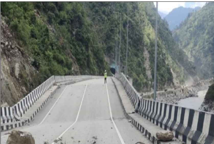
Photo 5 : Superstructure intact but piers settled. A boulder is on the carriageway.
