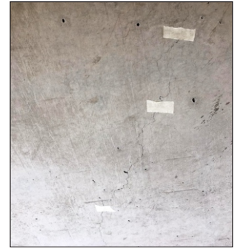
Photo 3: Closed View of Crack
