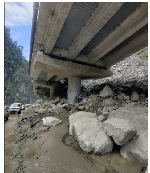
Photo 6 : Huge amount of debris on the pile caps. Two lane traffic on elevated road diverted to low level road.
