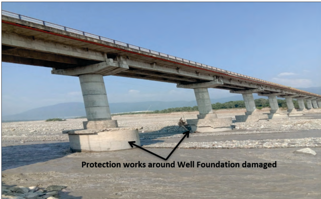
Fig. 5 : Exposed Well & Well Cap due to Scouring
