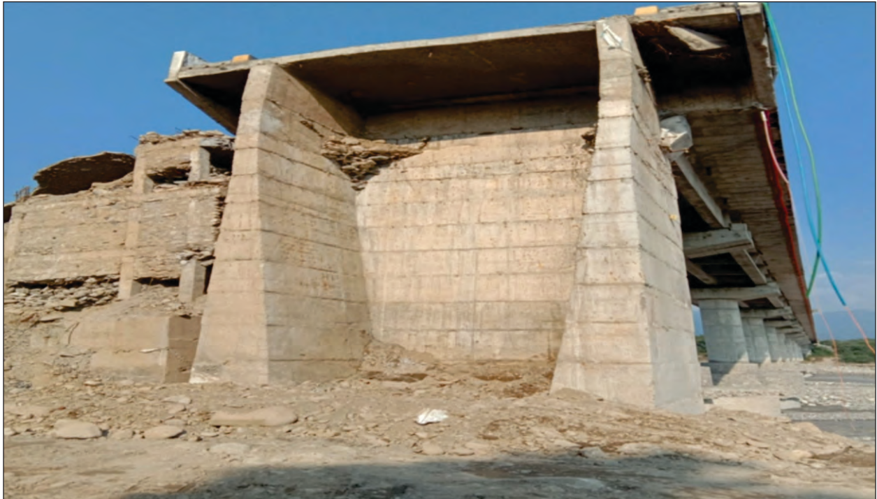
Fig. 3: Wash out Portion of Approach Road behind Abutment A1
