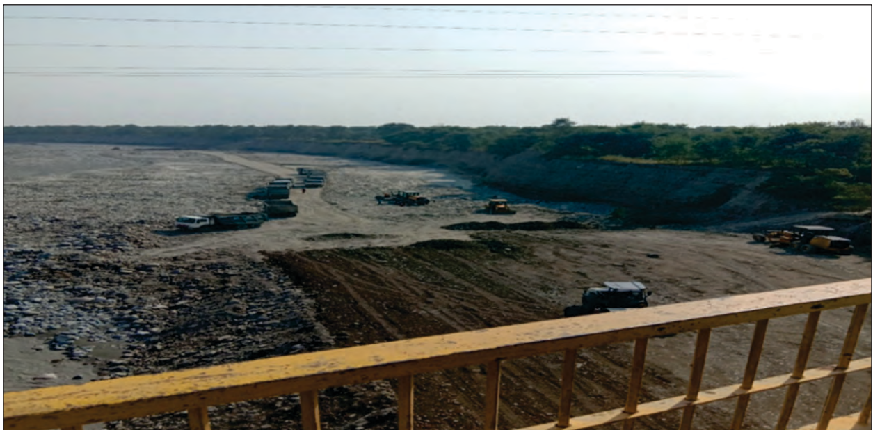
Fig. 4: Embankment Erosion on Down-Stream Side
