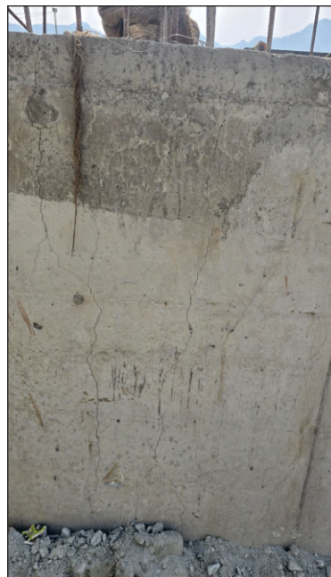
Photo - 02 : Cracks in false steining
