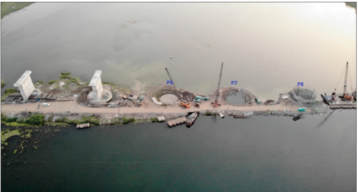
Photo-1 : View of Foundations affected due to presence of hard strata
