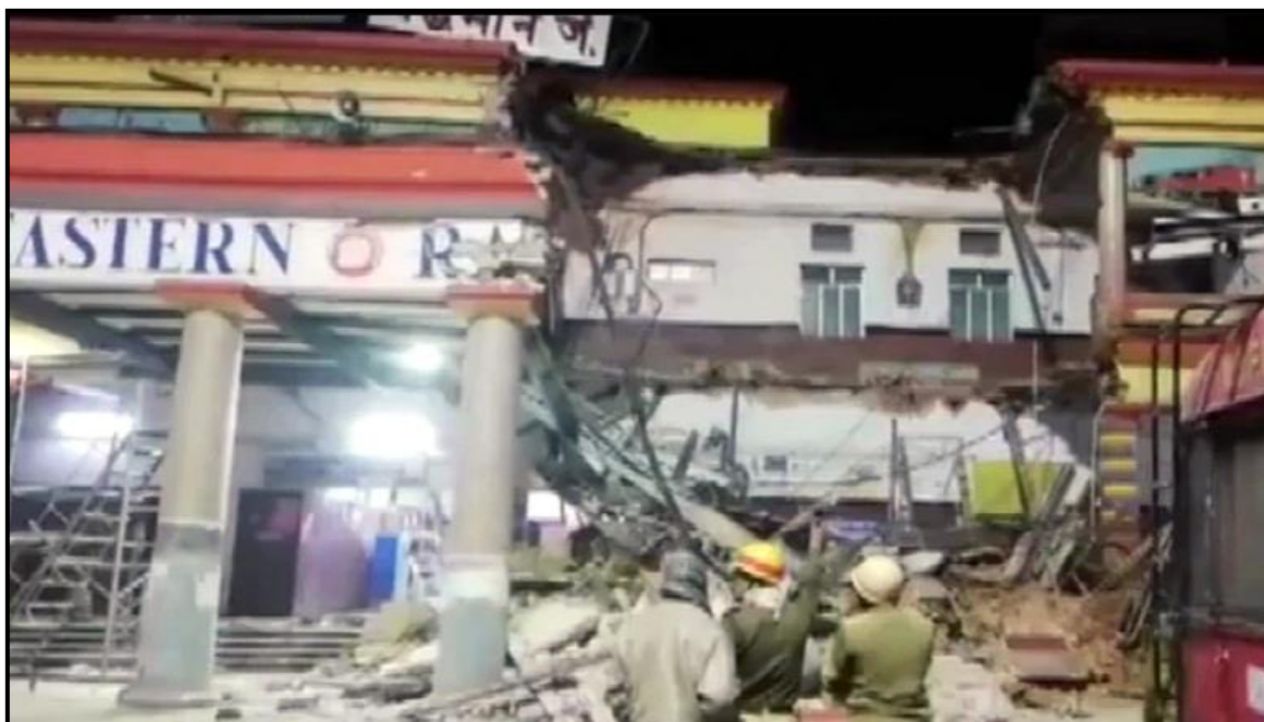
Fig.1:4th January,2020 - Collapse of the Burdwan Railway Station Building (Source: Internet)
