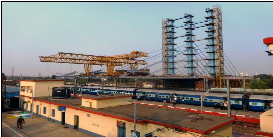
Fig.2: Four Lane state-of-the-art RoB in construction besides the Railway Station Building (completed in October, 2019)
