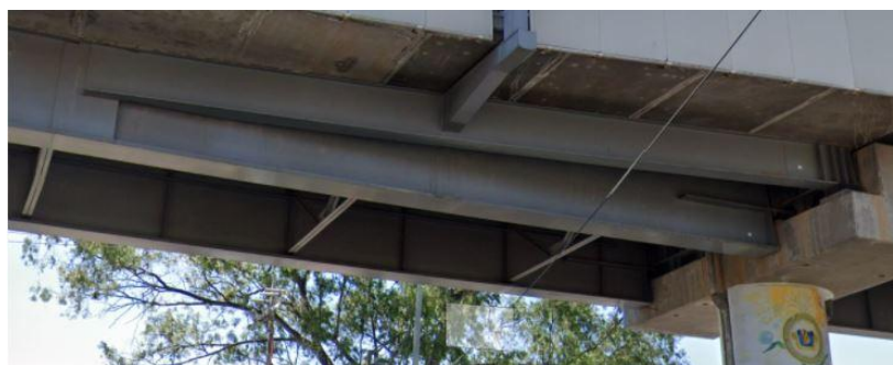
Fig. 8 A secondary beam attached to the main plate girder might have induced failure (Source: Ref.6)
